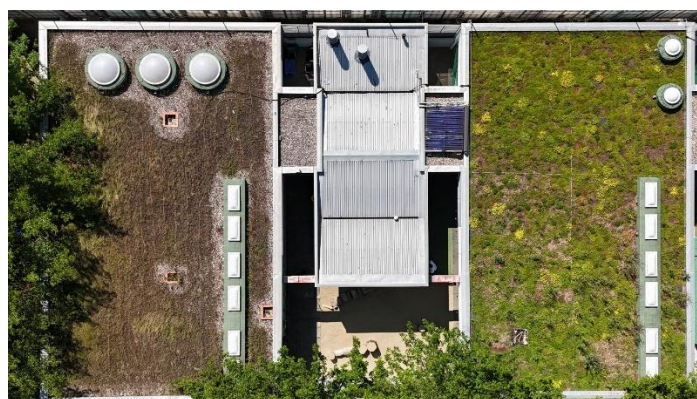
Fig. 1. Rooftop of the Ronda la Mercè Nursery School. Left side: original green roof as initially designed (failed implementation); right side: refurbished and fully functional green roof system
