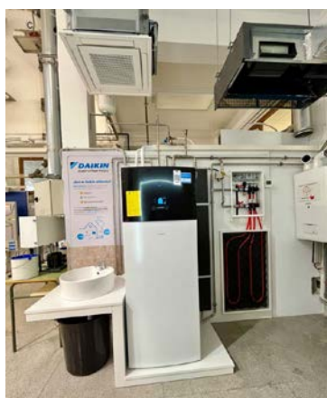
Imagen. Showroom Aerotermia DAIKIN.
